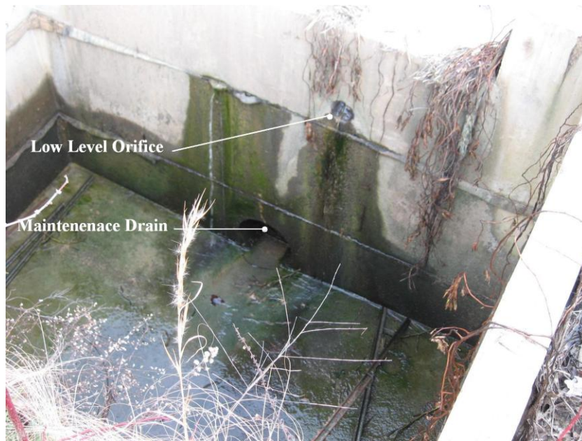
Figure 5.6 Draining Pond with Maintenance Valve
